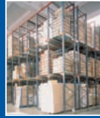
Drive-In Pallet Racking
